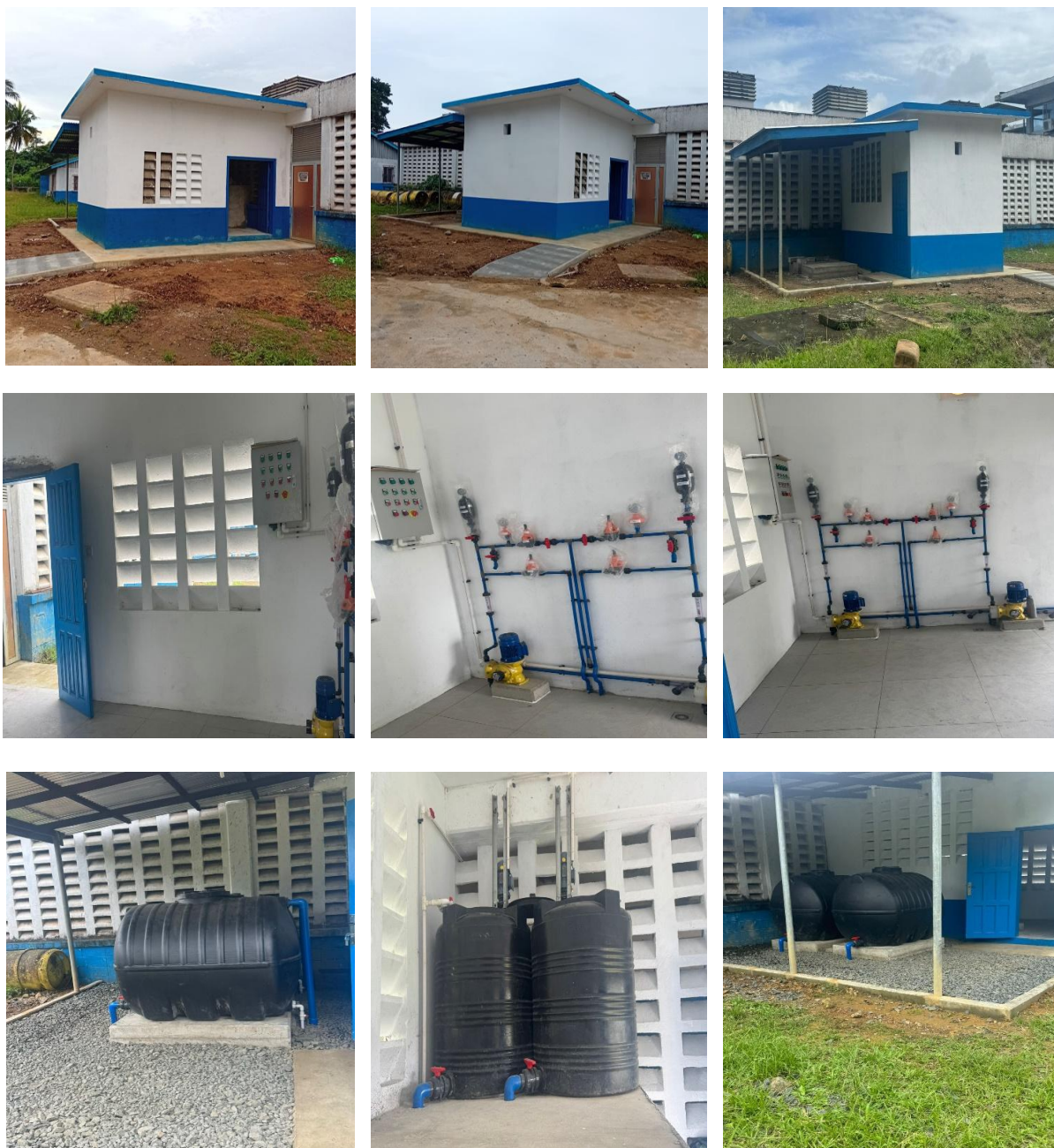
Figure 12: Chlorination and chlorine dosing systems at WTP
